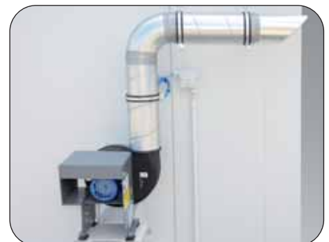
Ex-proof exhaust fan incl. exhaust air monitoring
