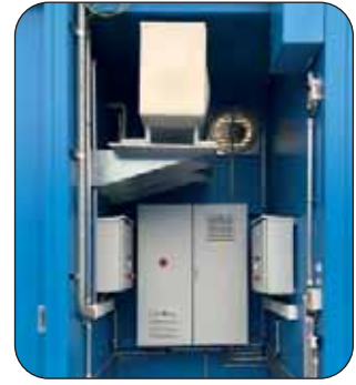
◆ Central control unit (control cabinet, sub-distribution, cooling unit)
