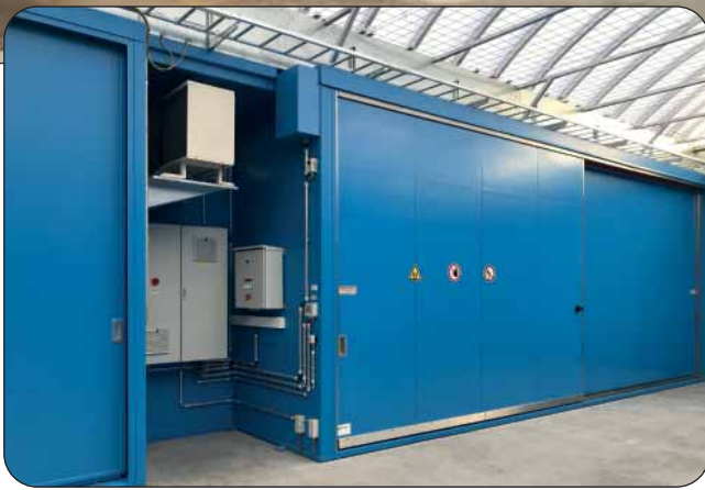
◆ Separate fire compartment with integrated fire protection container
