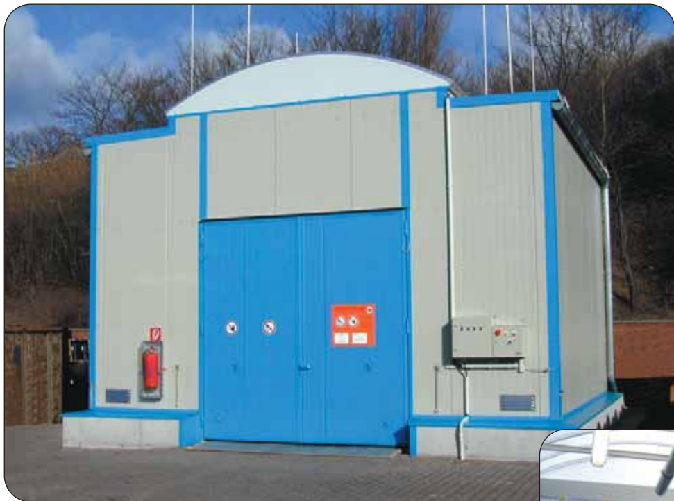
Operating equipment storage
