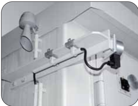
- Ex-proof exhaust air monitoring with signal horn - Door hold-open device
