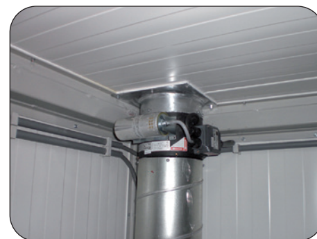
Air exhaust duct with K-90 shut-off device
